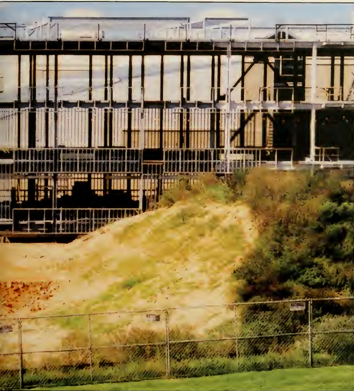
Under construction daily, the new physics and chemistry building is expected to be completed in 2005. Due to the increased participation in the sciences, the site behind ISAT was allotted as an addition to the previous science building, Miller Hall, located on the Quad.
